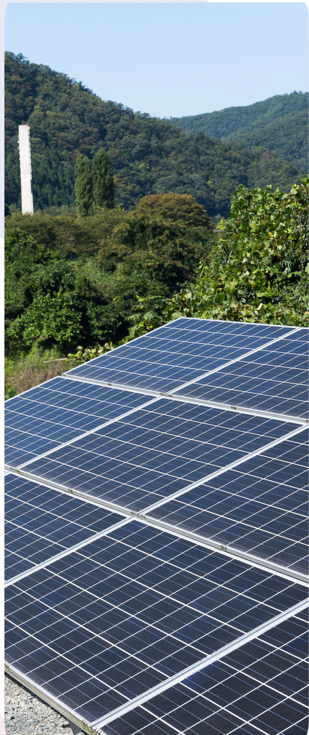
Stock Photo Of A Solar Plant
