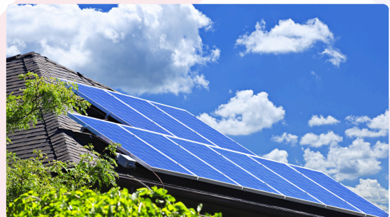
Stock Photo Of Solar Panels On Roof Top
